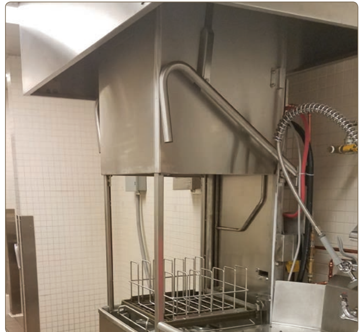
Dish room zone after scratch cooking.
