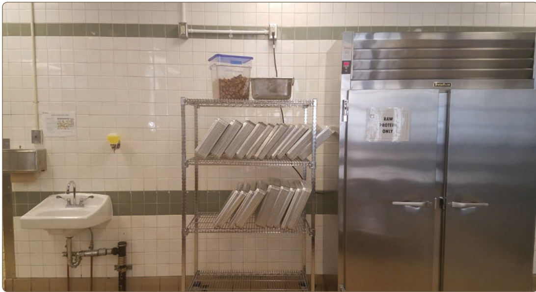
Installation of new handwashing sink and electrical for new raw protein reach-in refrigerator.
